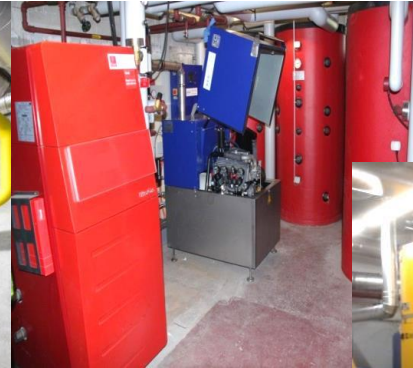
Mini-BHKW in MFH (Contracting)
